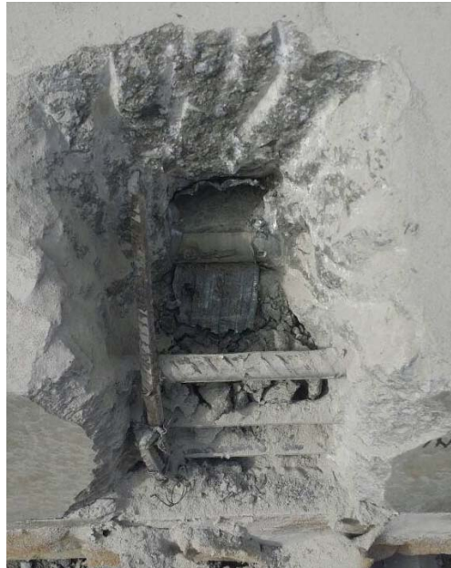
Photo of demolished area exposing sheath
