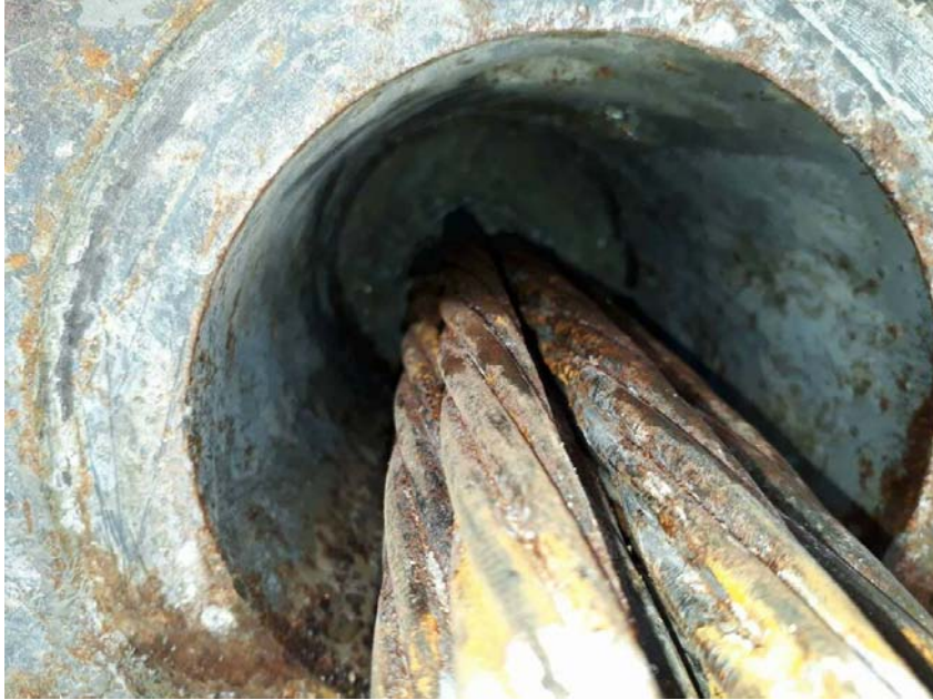
Photo of a blocked tendon in anchorage area
